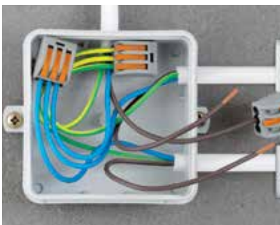
Wiring of flexible conductors in a junction box
